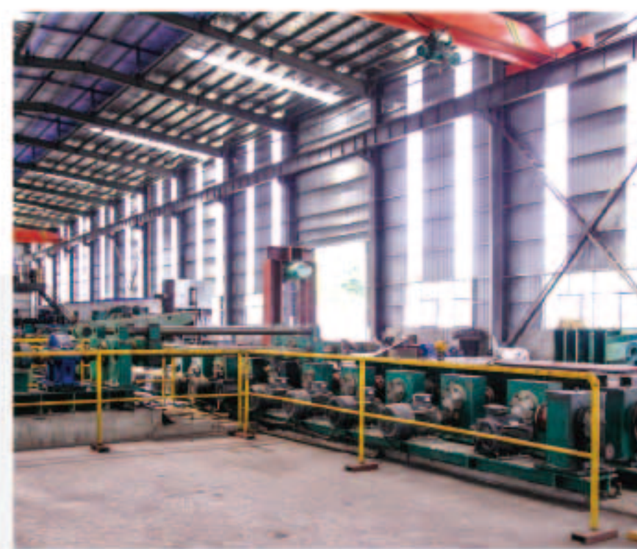
Hot Rolling Production Line
